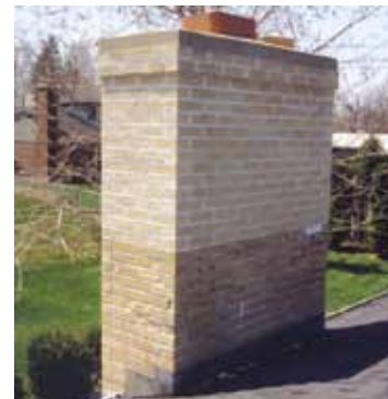
This partially rebuilt chimney would continue to deteriorate if left unprotected.
